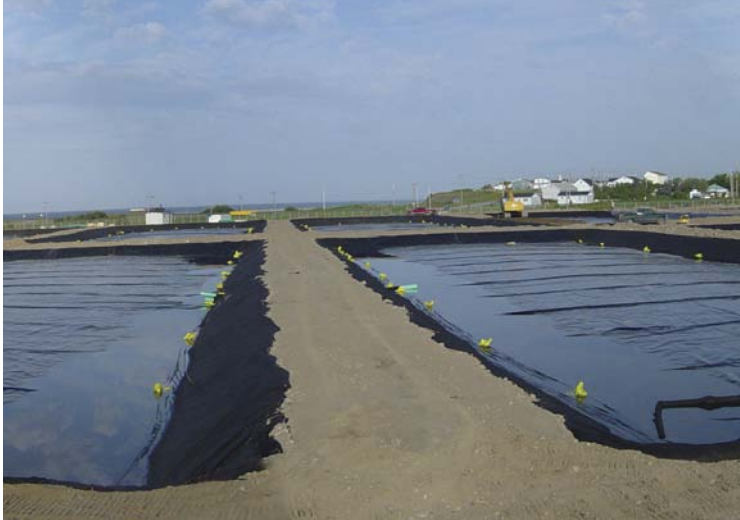
Biological wastewater-treatment beds are prepared as part of a chemical-free system for treating Stephenville's sewage (Photo: Town of Stephenville).
